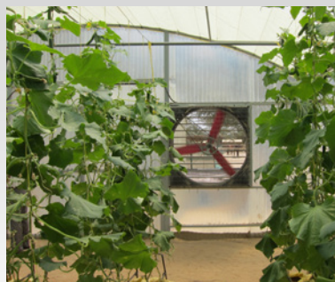
Galvanized Box Fan in greenhouse
