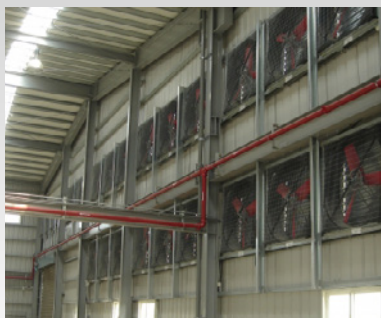
Galvanized Box Fan in industry
