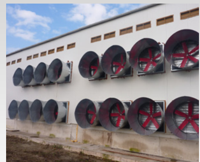
Galvanized Cone Fan in poultry house
